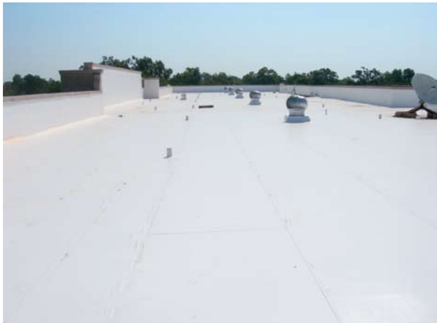
■ Duro-Last custom designs each roof based on the layout and penetrations. (Photo courtesy of Mid-Western Commercial Roofers Inc.)
